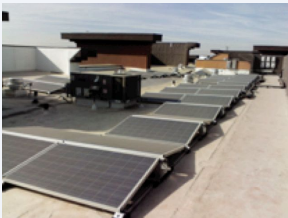
60 Rooftop Panels (42 with SunDrum Collectors)
