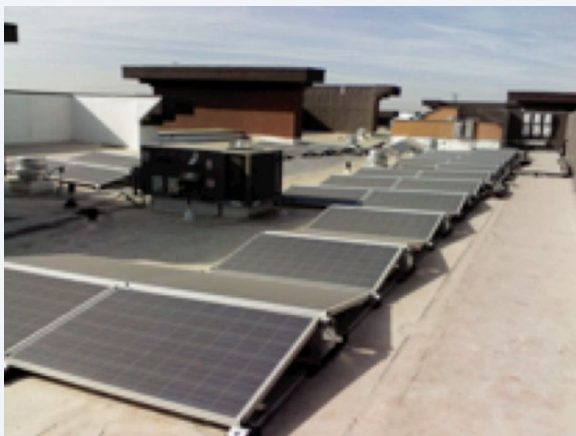
60 Rooftop Panels (42 with SunDrum Collectors)
