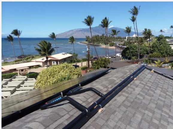
Rooftop Solar Panels
