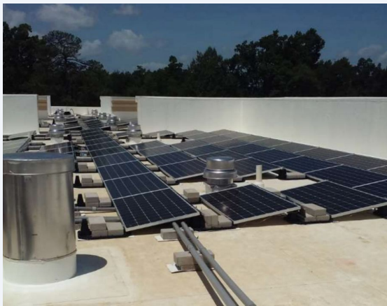
Rooftop Solar Array
