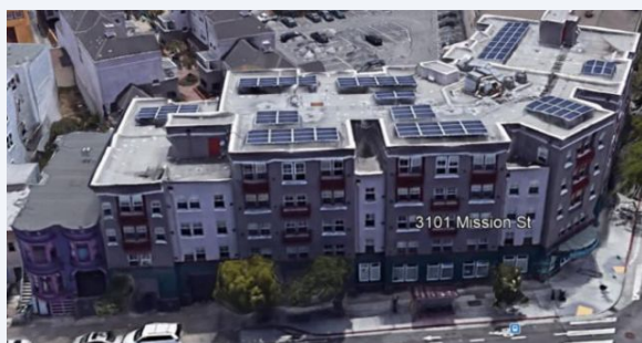
SunDrum Mounted Under Existing PV
